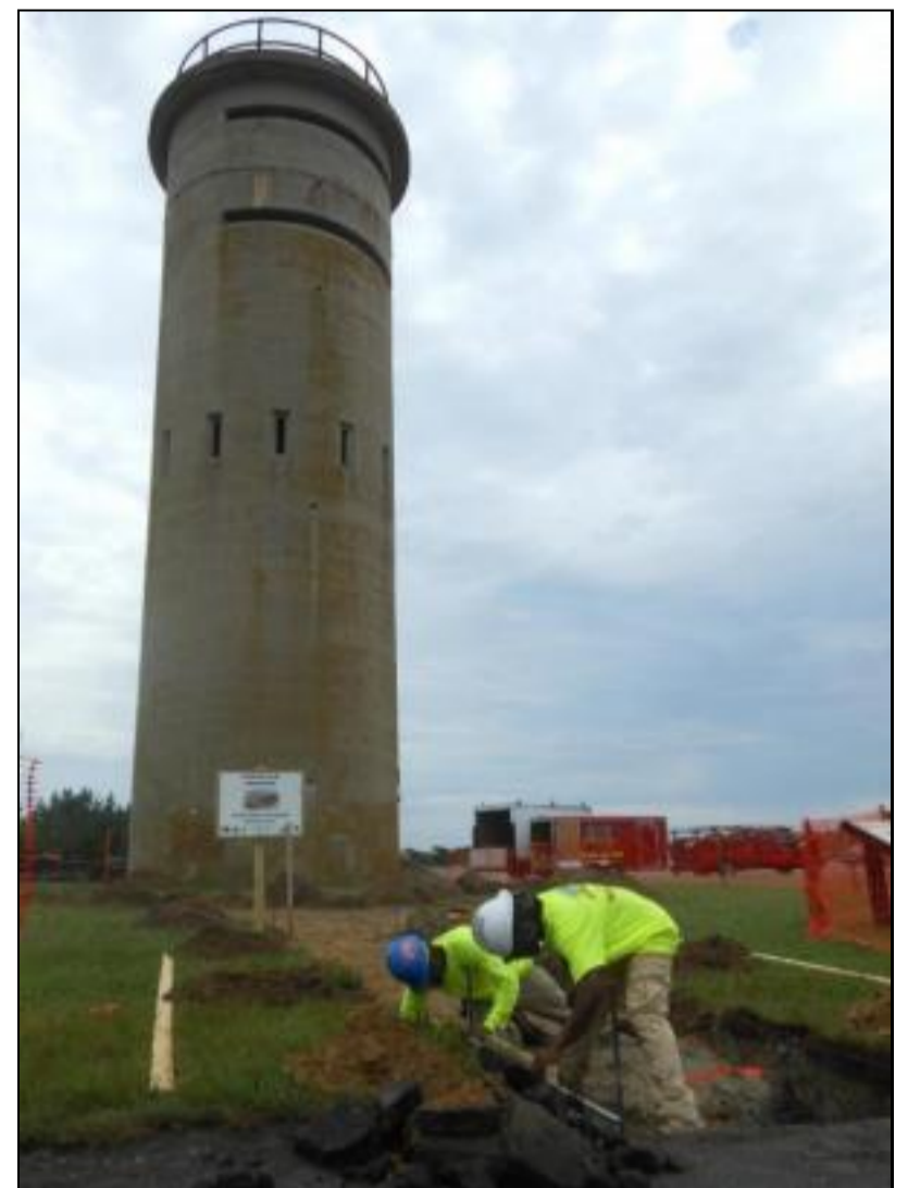
Kent Construction's Ron Summers and Mike Derrickson run a string before work can begin on a new sidewalk. CHRIS FLOOD PHOTO
