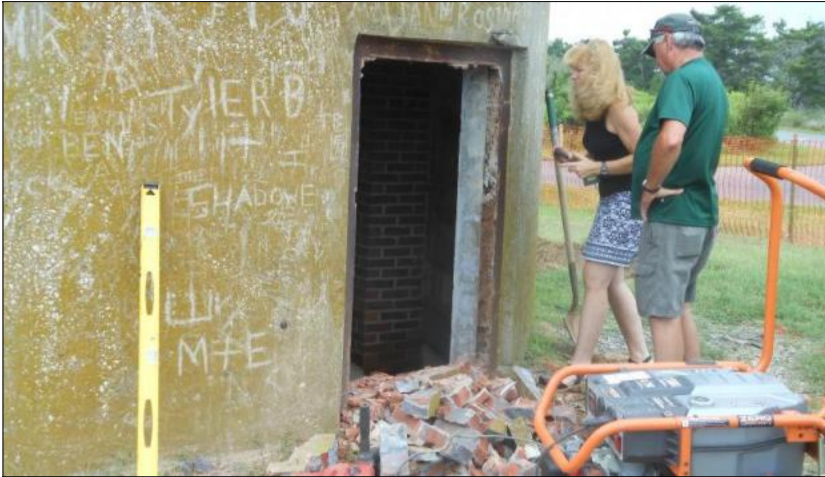
A pile of bricks lies at the feet of Cindy Todd, construction project administrator for Delaware State Parks, and Pierce Thompson, site manager for the division, as they look at the condition of the tower at Tower Road. CHRIS FLOOD PHOTO
